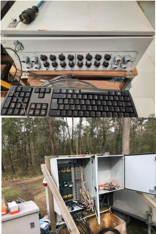
Customized heating system and cabinet
